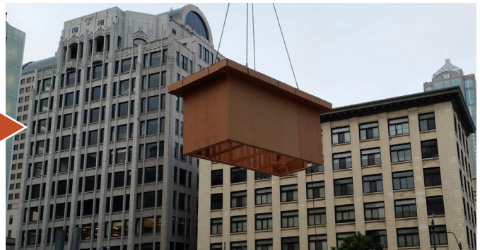
The sump pit formwork is delivered to the project site 'just-in-time' for the concrete pour.
