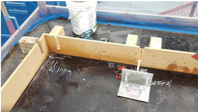
The formwork arrives on site as an easy to assemble 'kit-of-parts' that requires smaller field crews to install and simplifies the work.
